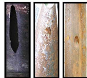
Flaws Shown Above From Left To Right Rod Wear Split, Internal Pitting, Pitting With Hole
